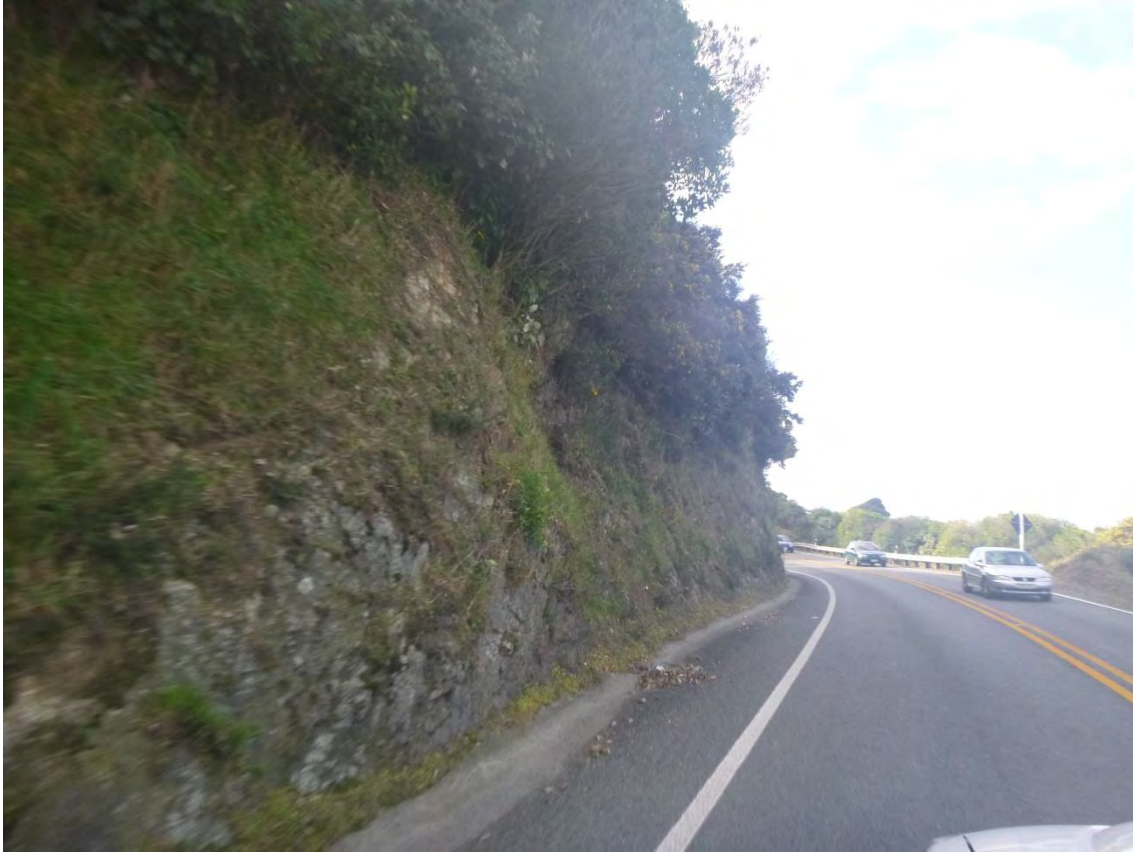
Photo 1: Steep cliff bank, horizontal curve, limited sight distance, heading west
