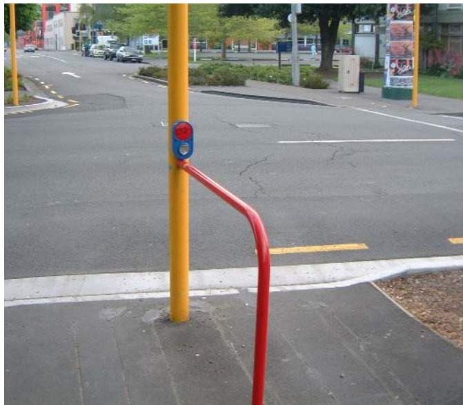
An example of an automatic bicycle detector call box, Christchurch, with detector loops underneath
